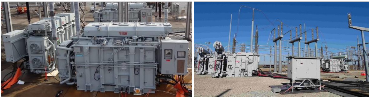
Figure 5 - Rapid recovery resilience transformers on site (Case I and II) (photo: Siemens)
