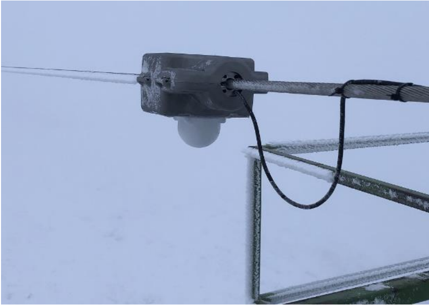
Fig. 10: Ampacimon™ vibration-based sensor [9] installed on single conductor (Conductor : ACSR LA-180, span length: 190 [m]) at Dead Water Fell test site (owner : EA Technology [21]) Sensor has been installed during a period with some deposit on conductor. Snow has been cleaned up close to sensor location for installation purpose (no snow in front of the sensor and snow behind sensor).
