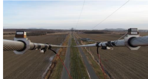
Figure 7 Accelerometers near tower 2 to measure aeolian vibrations
