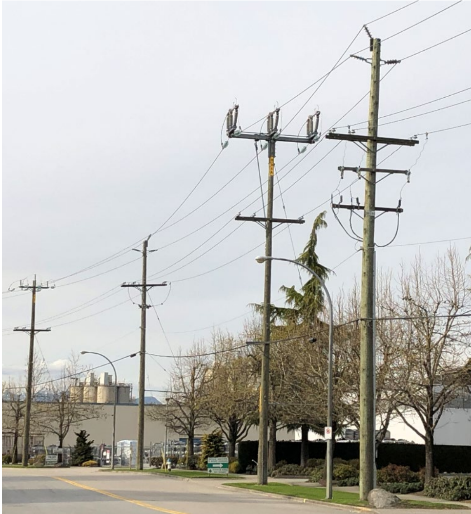
Figure 8. Photo showing the tap portion of a 69kV tap connection.
