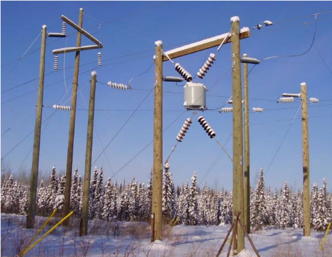
Figure 7. Photo showing an example 138kV wave trap structure.
