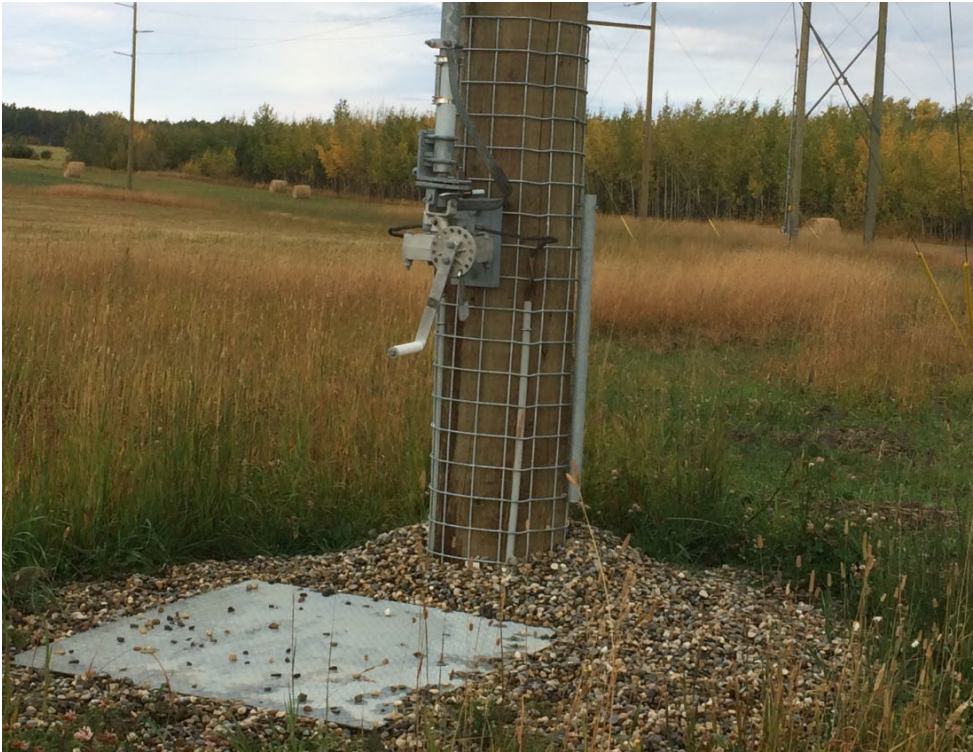
Figure 6. Photo showing an example of grounding for a 138kV disconnect switch structure.
