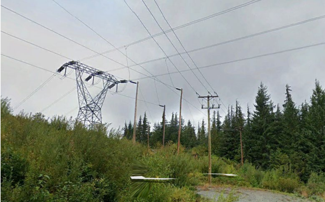
Figure 5. Photo showing an example of 230kV flying tap connection.
